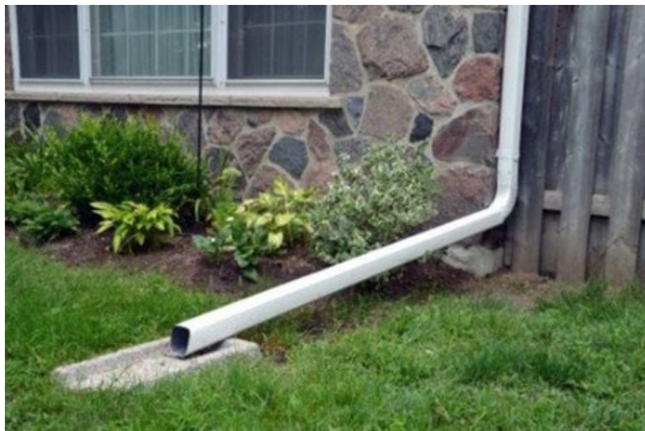
Figure 4.9. Disconnected Downspout to a Pervious Surface
